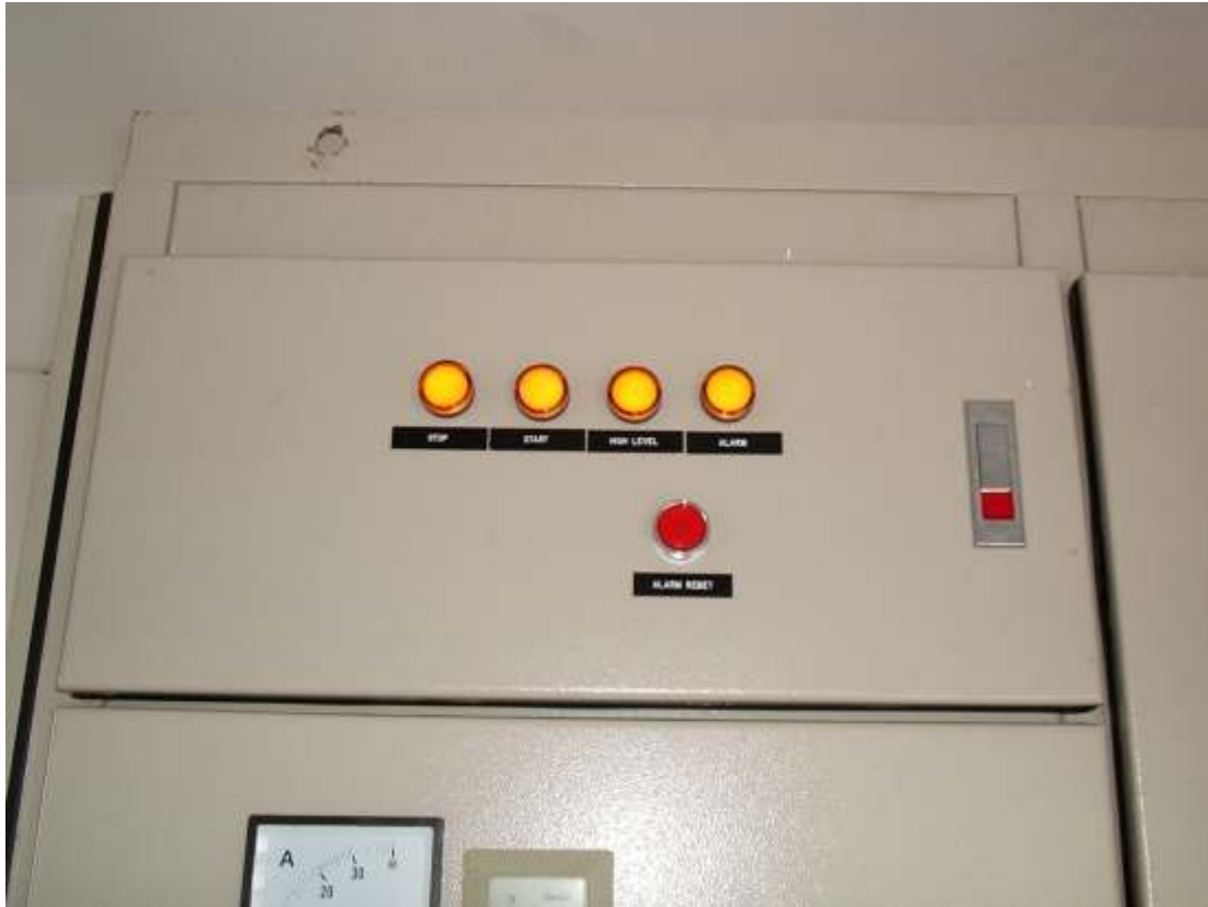
Fig 7 Level Control Switches Compartment
