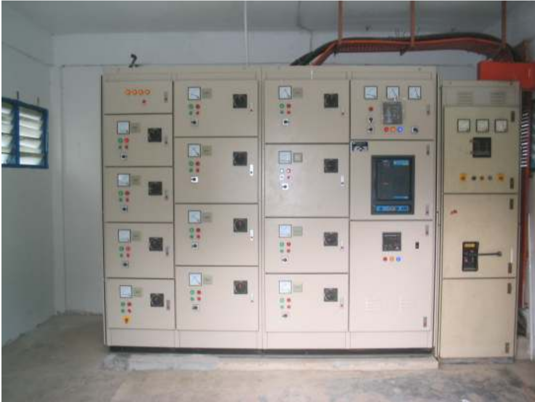
Fig. 6 New Motor Control Centre
