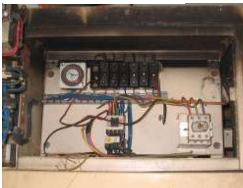
Fig. 2 Damaged MCC panel
