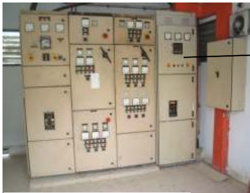
Fig. 1 Existing MCC panel
